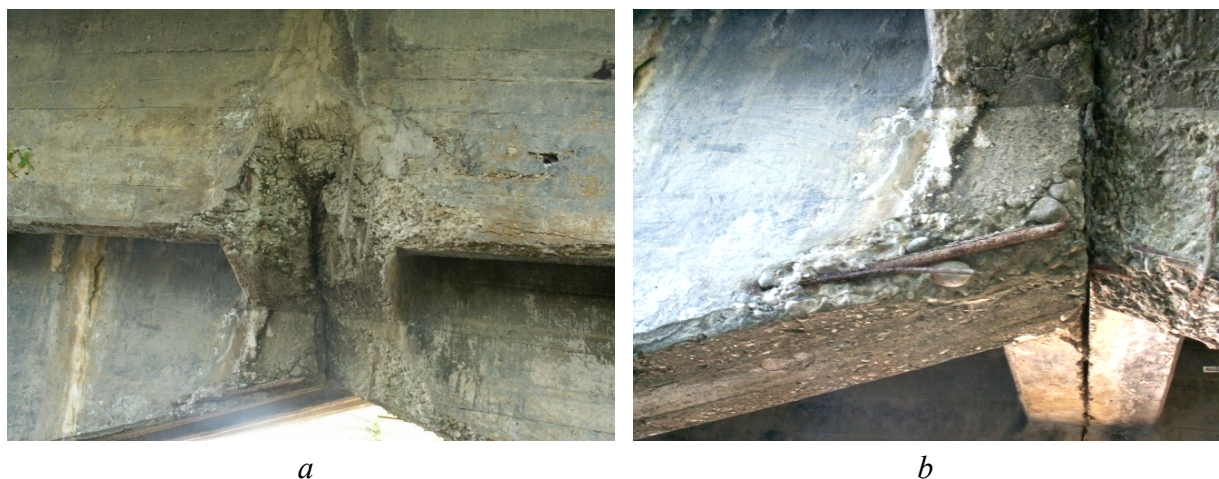
a – вид стыка между первым и вторым отсеками снаружи, слева видны кальцитовые натеки; b – вид с запада на стык первого и второго отсеков, разрушен бетон, обнажена и корродирована арматура a – view of the joint between the first and second compartments from the outside, calcite deposits are visible on the left; b – view from the west at the junction of the first and second compartments, the concrete is destroyed, the reinforcement is exposed and corroded
